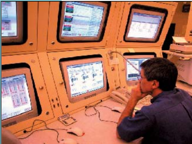
The control room's original analog control systems have been replaced by a digital control system, using PCs and PLCs to run all Weston operations.
