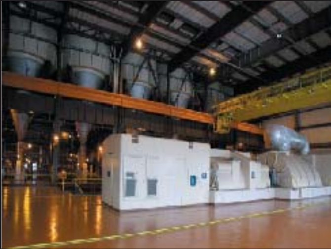
A massive turbine engine (center) generates electricity. The steam condensate return is on the right. To the left is the exciter that controls voltage and the amperage of the output.
